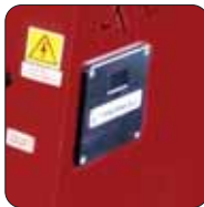
Manuel Control Panel
